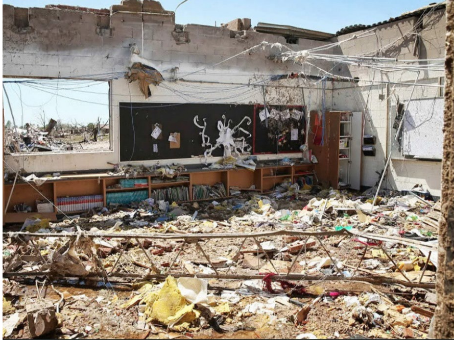
Figure 3: Damages at Plaza Tower Elementary
